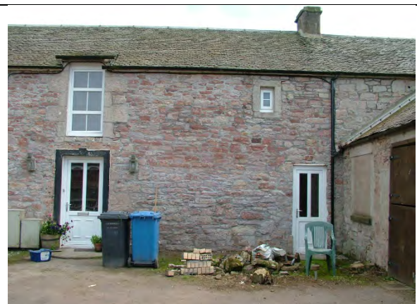
Plate 2. Showing west end of north wall with original upper floor window and also slit window between two doors.
