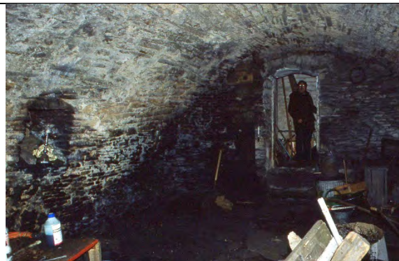
Plate 18. Showing the barrel-vaulted basement looking west to the entrance and stair on left side
